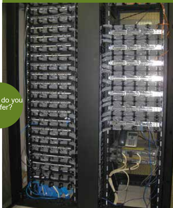
After using Ausrack Plus cable management system
